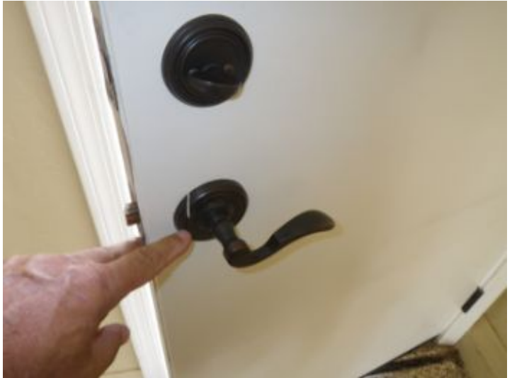
Garage exterior door knob needs adjustments
