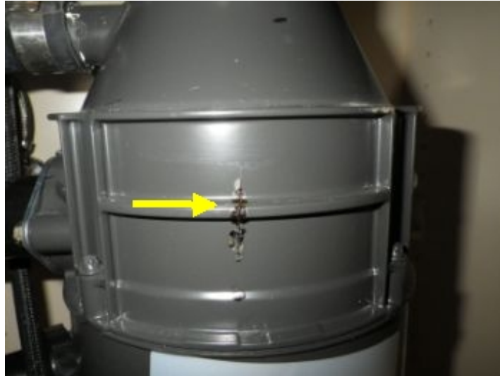
Garbage Disposal is corroded and should be replaced before it leaks or fails.
