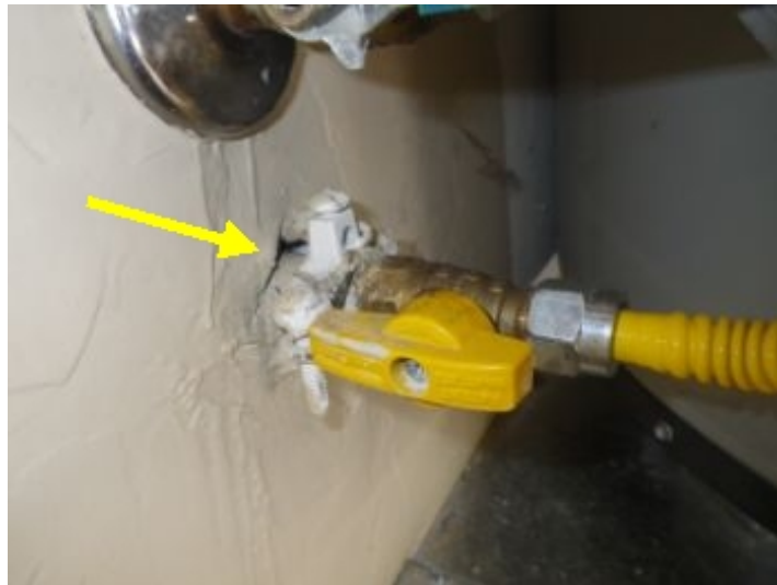
Bond wire visible at gas piping
