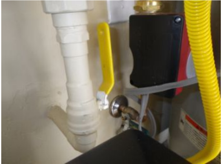
Water shut off in the garage, excellent
