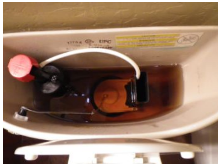
See note in General Plumbing section on Rusty water
