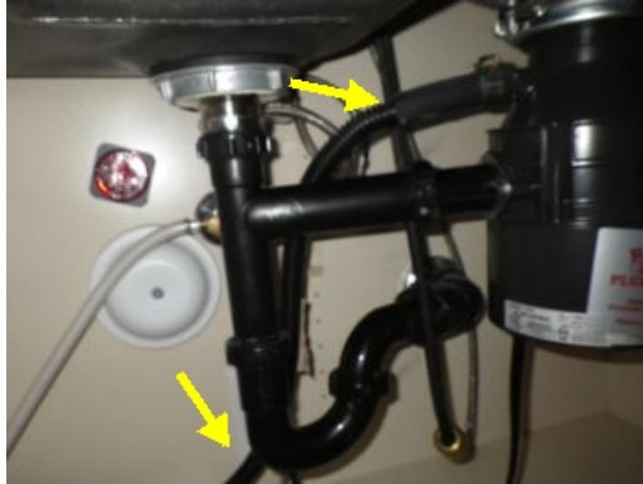
Cross connection- Lack of a proper high loop or air gap noted at dishwasher drain line.
