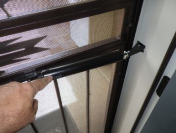
Entry screen door self closer needs adjustments or replacing to operate correctly
