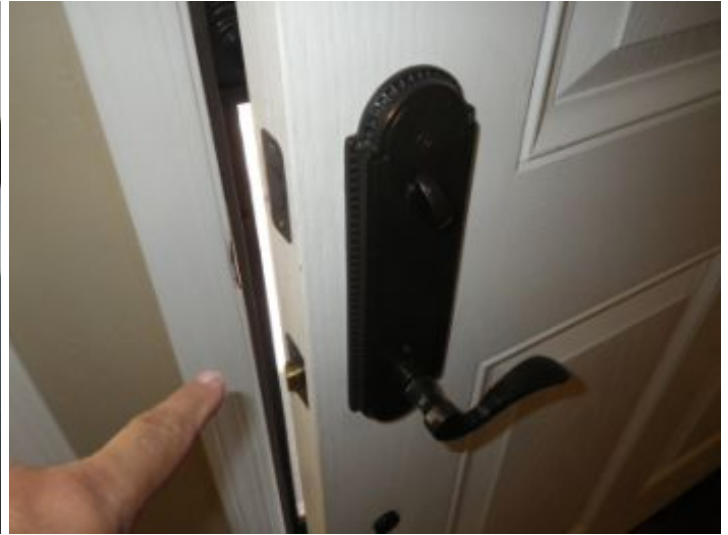
Front door does not latch, recommend adjustments for safety
