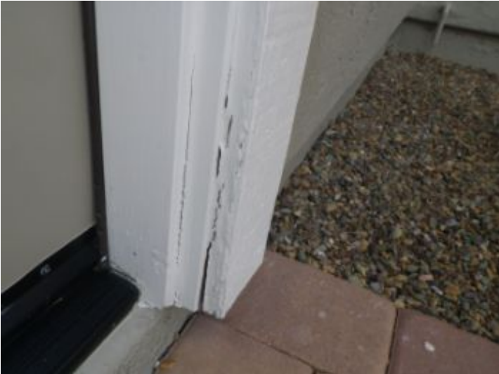
Recommend caulking and re painting the lower section of rear exterior garage jamb
